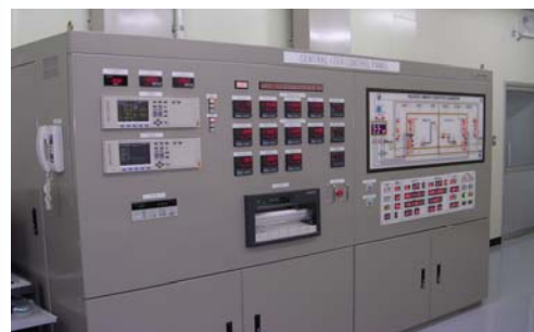
Calorimeter Control Panel
