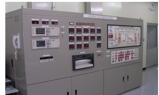
Calorimeter Control Panel
