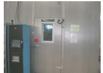
Temperature & Humidity chamber for Air-conditioner (IEC 60335-2-40) Maximum load : 48000 Btu / hr
